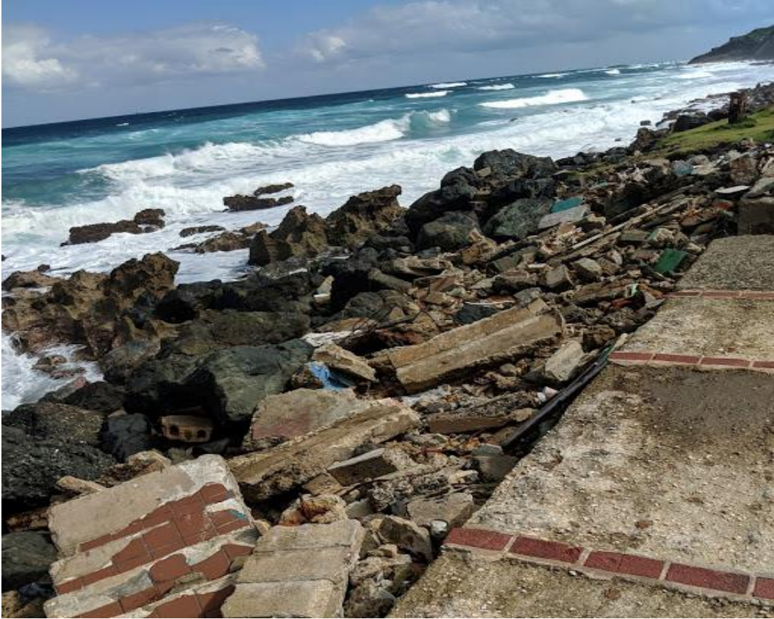
Figure 3.3 Tidal Surge Damage
