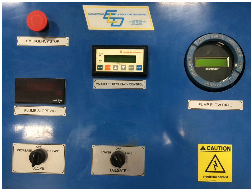
Figure 3.2. Flume control panel featuring digital displays and adjustment toggles.
