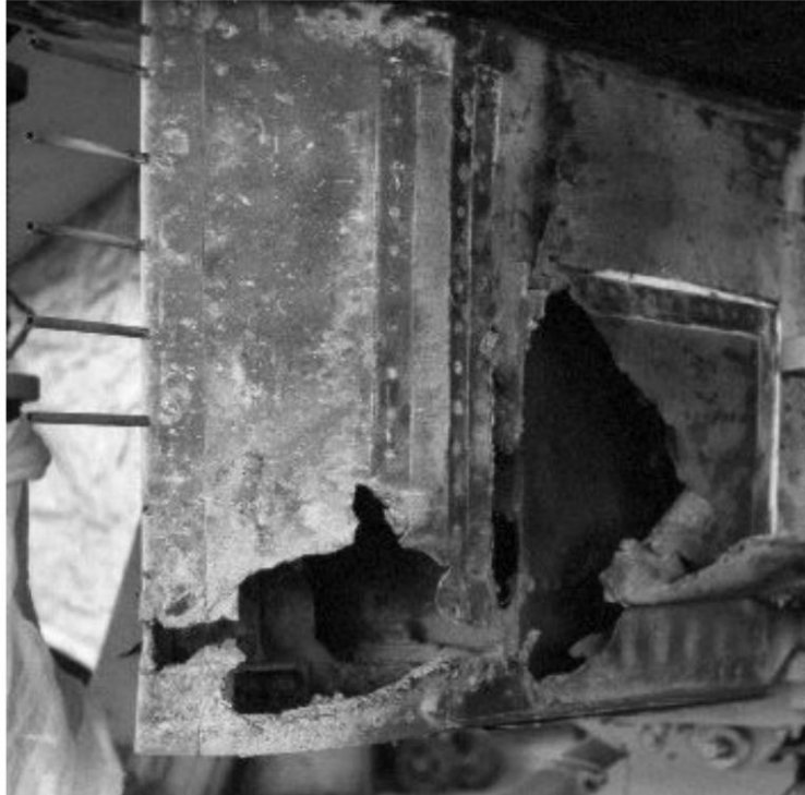
Figure 6: Pylon Damage on the X-15 Caused by Shock Shock Interactions [22]
