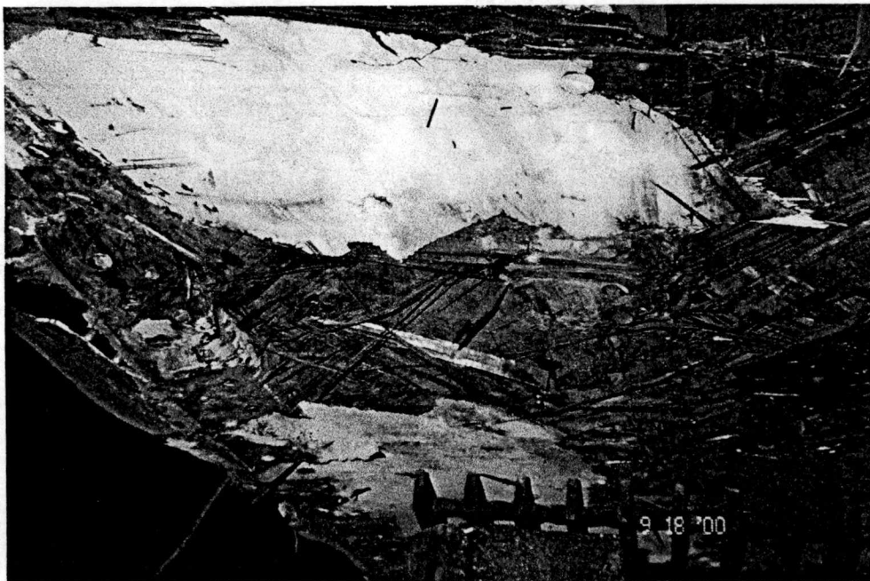
Figure B-21 Fire Damaged Composite Material Showing Multiple Levels of Burn Damage.
