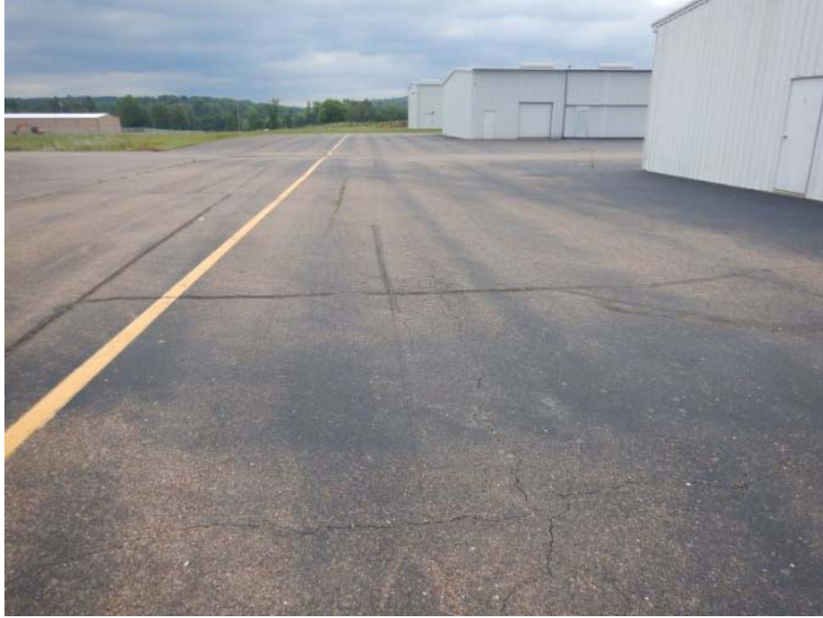
Figure 10. TH01SA-001 pavement photo L&T Cracking
