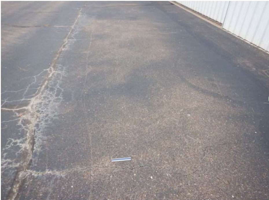
Figure 11. TH01SA-001 pavement photo Alligator Cracking
