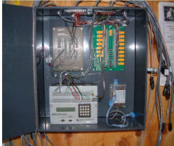
Figure 2.2 Data Acquisition Equipment in PVC Enclosure.
