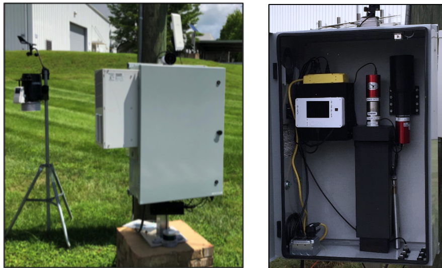
Figure 22: Image of a node ( left ) on the ORNL sensor array along with an image inside the enclosure ( right ).
