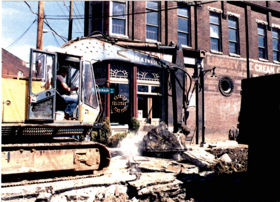
Figure 5.3 - Sidewalk Demolition on East Jackson Avenue Photo Credit: George Scott, Old City Mercantile
