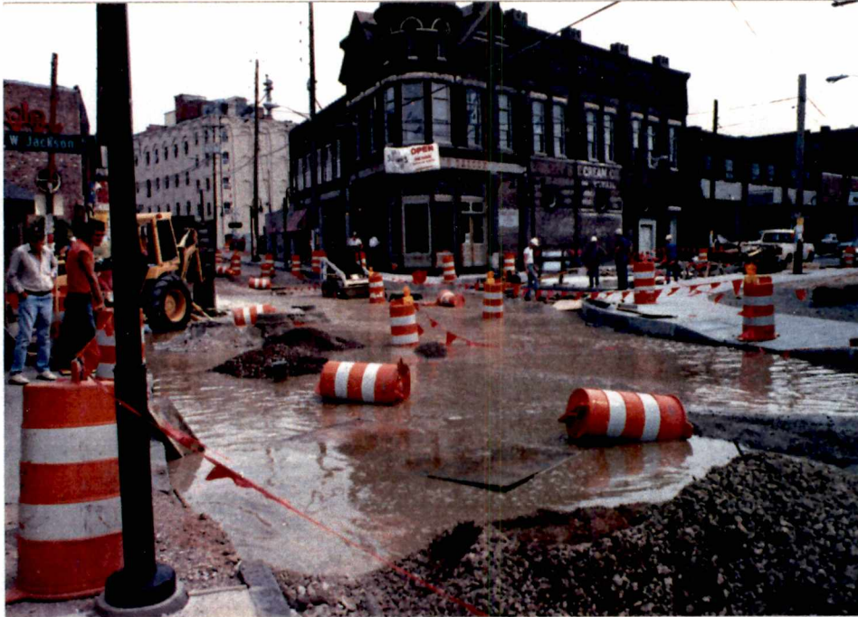
Figure 5.5 - Intersection Construction, Jackson and Central Photo Credit: George Scott, Old City Mercantile
