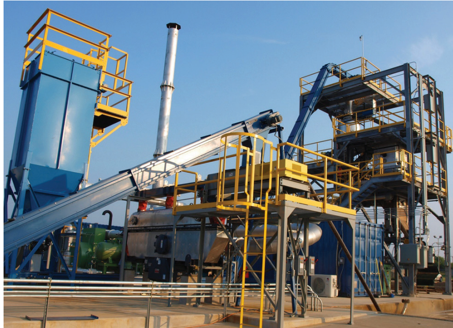
▲ The Lebanon plant will be similar to the gasification plant in Covington.
