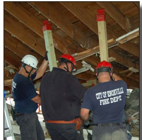
(Right) Another team uses taller posts to shore up another side of the structure.
