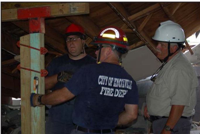
Walter Idol, right, instructs the group that has tunneled in how to add posts near the back of the collapsed building.
