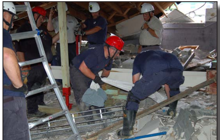
After securing the structure and lifting a large metal beam, the firemen free a "victim" from the destruction.
