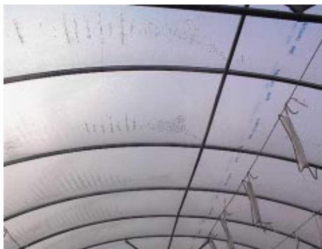
Condensation problems caused by excessive humidity levels.
