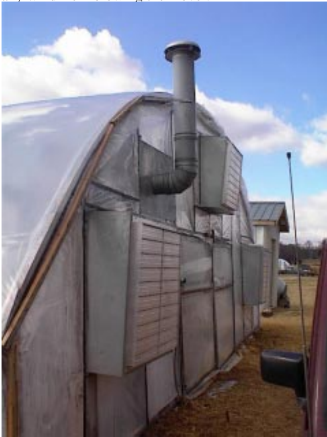
Vented heater exhaust stack
