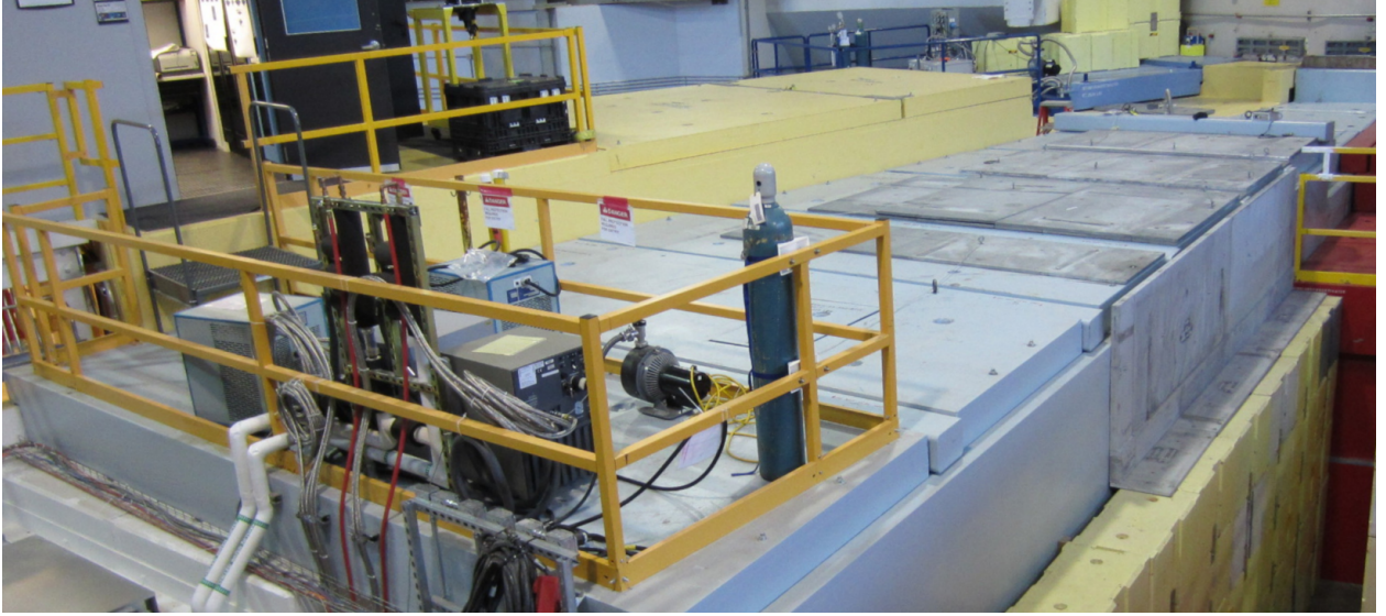
Figure 3.6: A view of the Beamline 13 radiological shielding.
