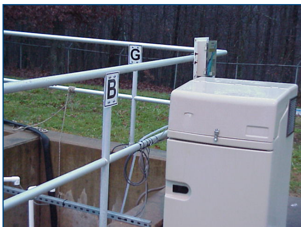
Effluent composite sampler and grab sample locations marked on a chlorine contact chamber.
