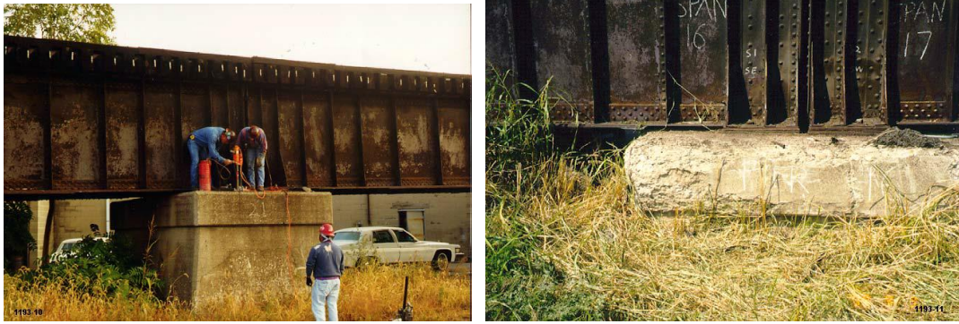
Figure 3.6 Typical Pier Condition in Cincinnati Bridge (Uppal et al. 2000)
