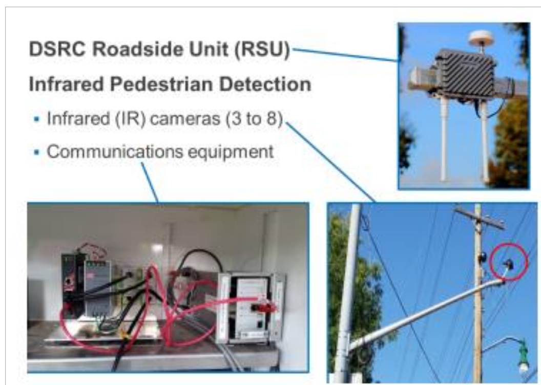
Figure 2.4 Infrastructure Subsystem-Roadside Units (RSU)
