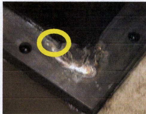
Figure 14. Another leakage area
