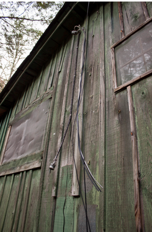
Homes in disrepair Images by J. Wessels, 2014
