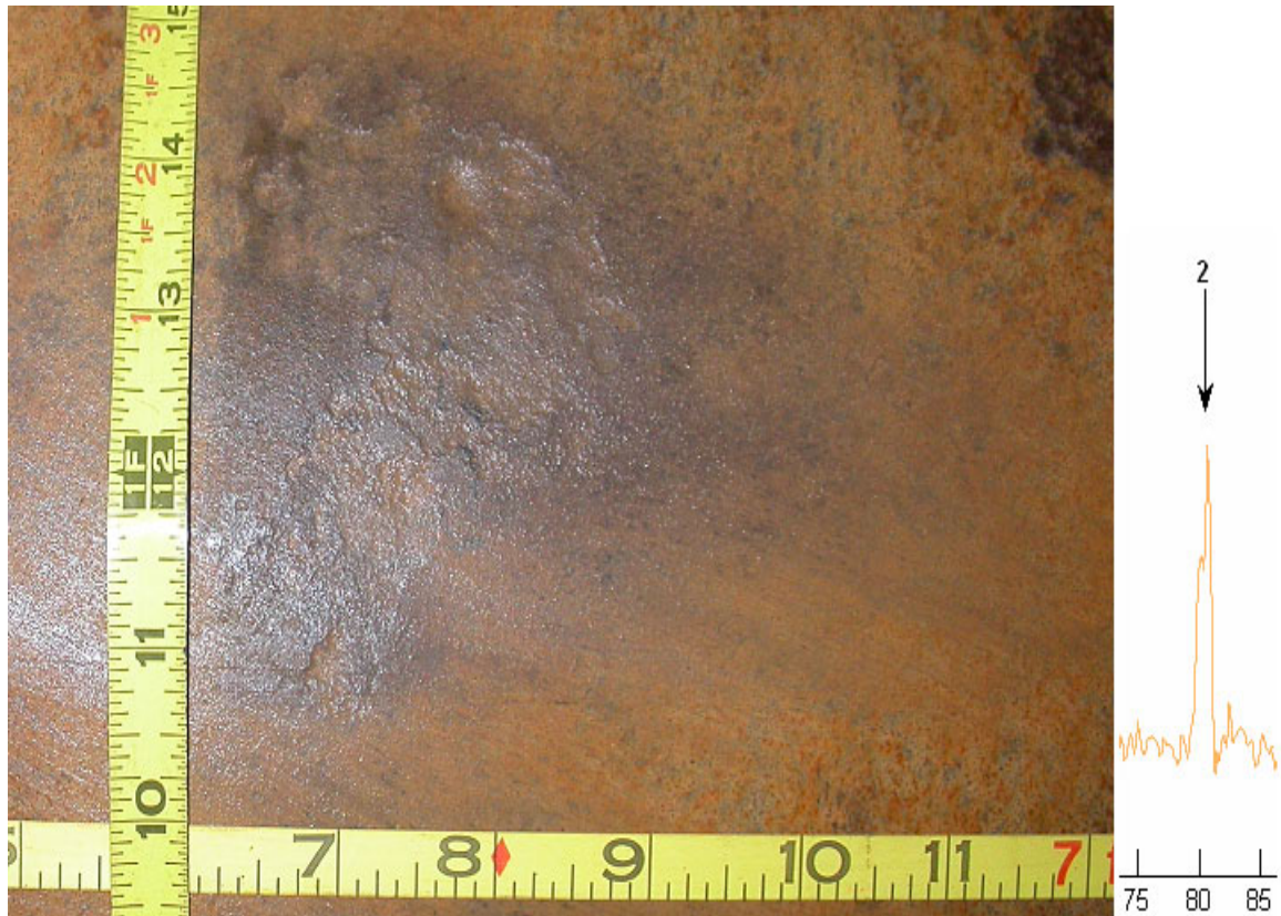
Figure 4.15: Indicator: Arrow 2; Defect Type: Corrosion
