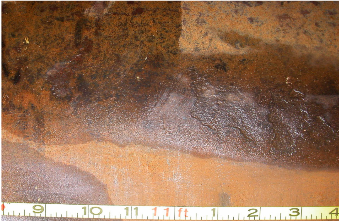
Figure 4.21: Indicator: Arrow 6; Defect Type: Corrosion
