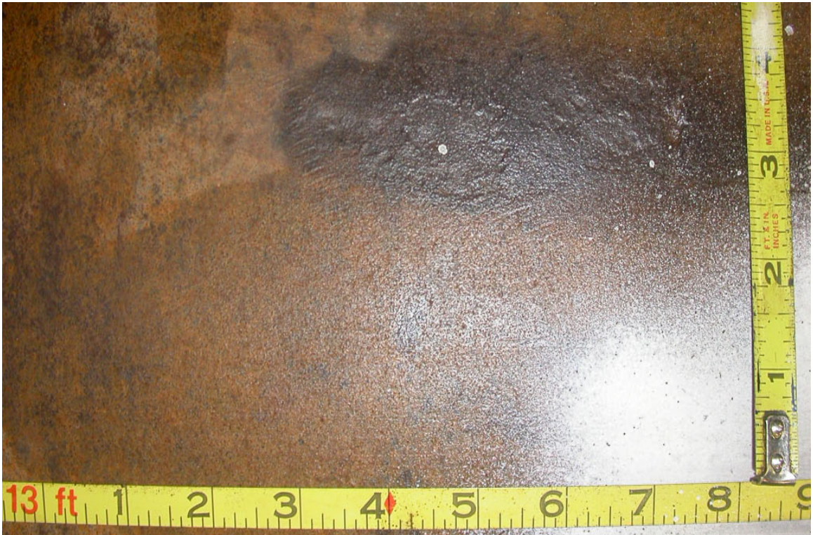
Figure 4.23: Indicator: Arrow 7; Defect Type: Corrosion Patch
