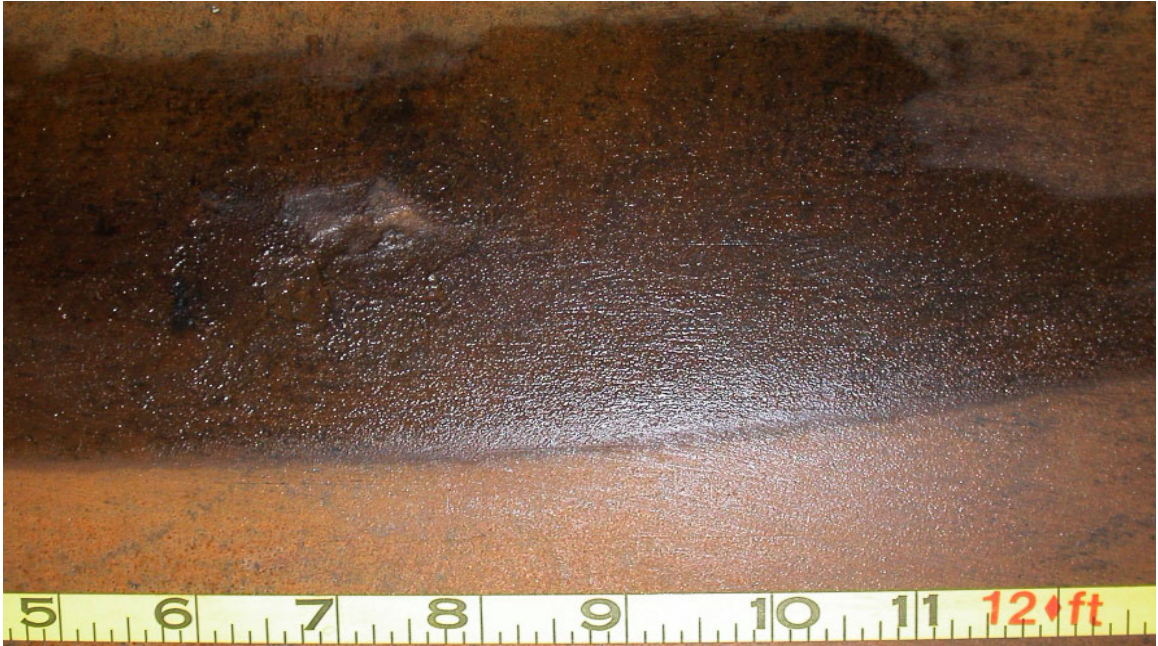
Figure 4.22: Indicator: Arrow 6; Defect Type: Corrosion
