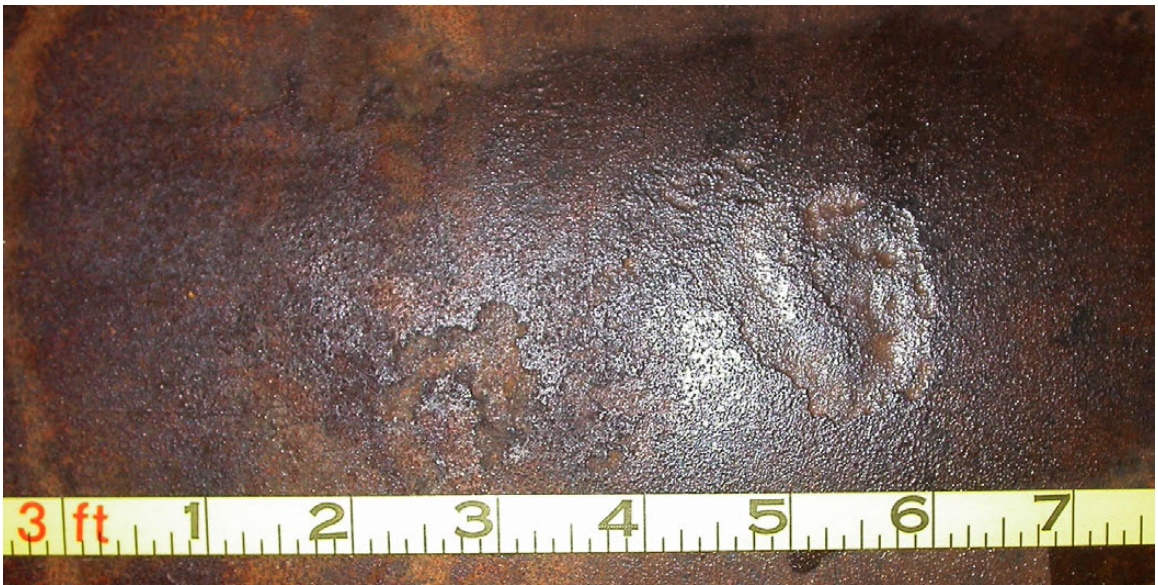
Figure 4.14: Indicator: Arrow 1; Defect Type: Corrosion
