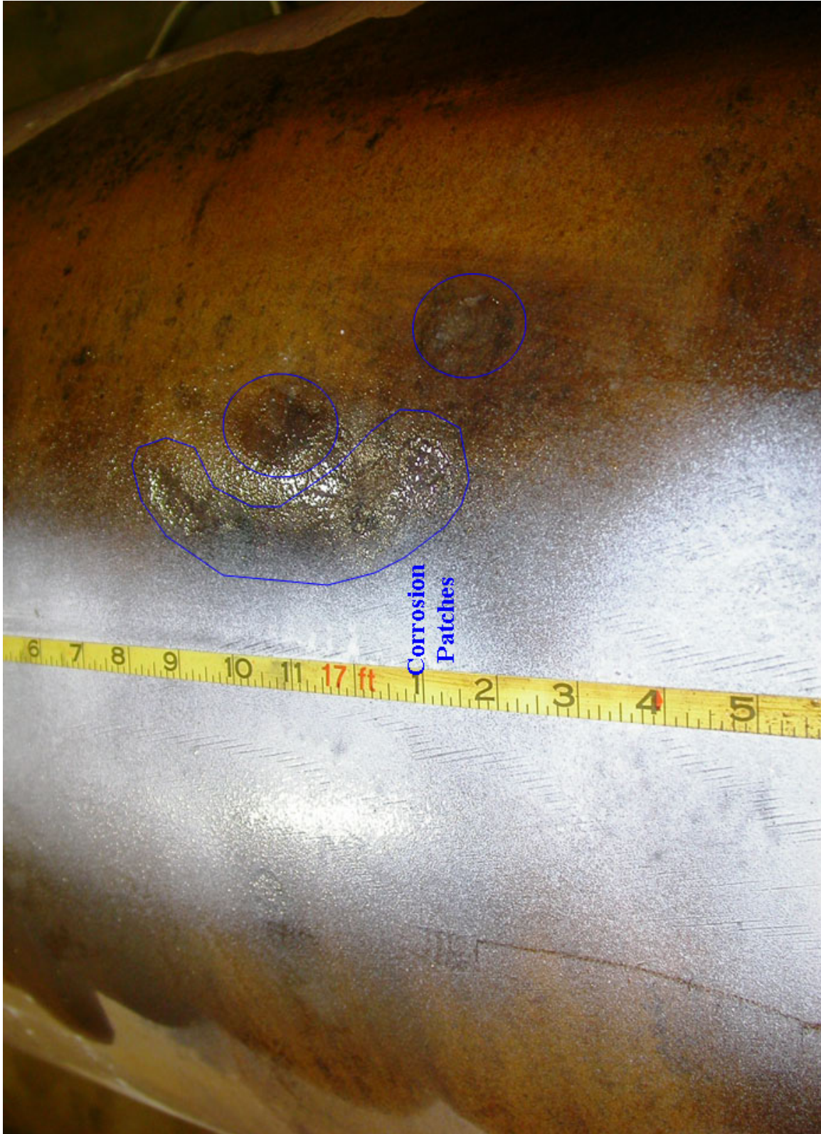
Figure 4.25: Indicator: Arrow 8; Defect Type: Corrosion Patches
