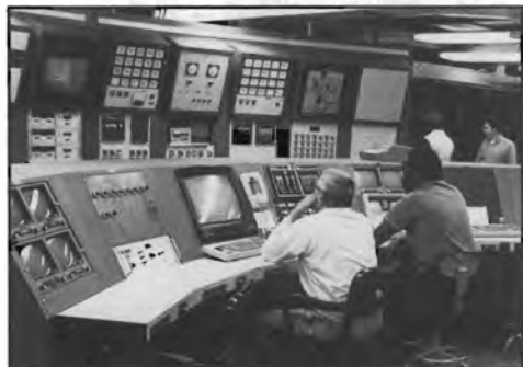
The control room of the Coal Fired Flow Facility at UTSI.
