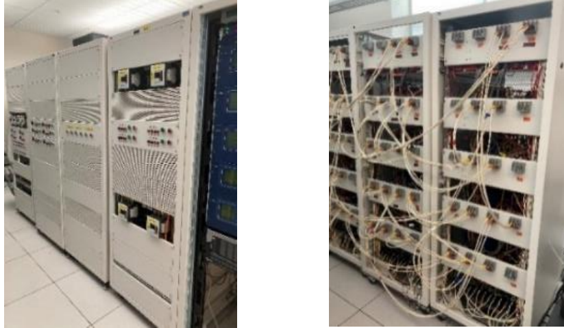
Figure 3-10 6-converter system based on HTB: converter cabinets (left) and variable inductor cabinets(right)
