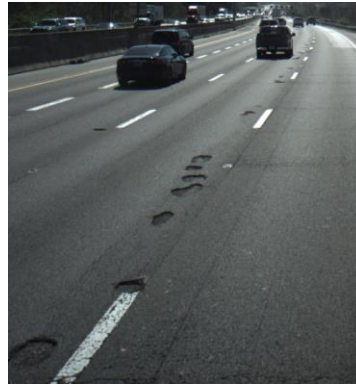
b. Pothole zone
