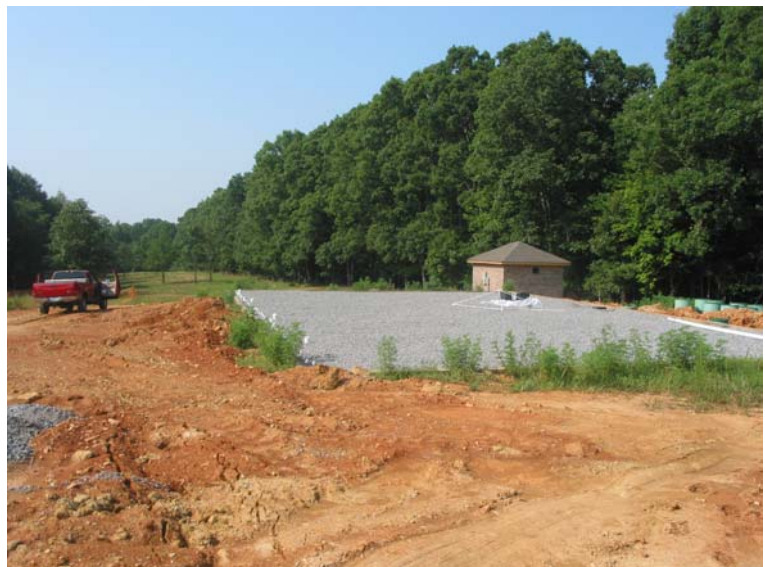
A recirculating sand filter and subsurface drip field. The drip field is in the background. This wastewater treatment system can handle 20,000 gallons per day.
