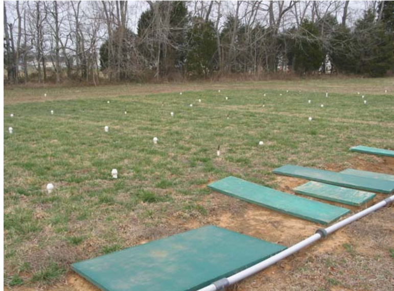
A wastewater subsurface drip irrigation research site. Shown in the picture are samplers that are used to take soil moisture samples. It just goes to prove that the grass is greener over the septic system
