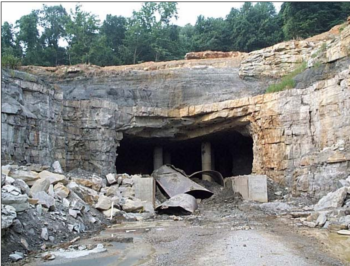
Figure 16. Fort Hartford Mine Superfund Site “A” Portal Landslide
