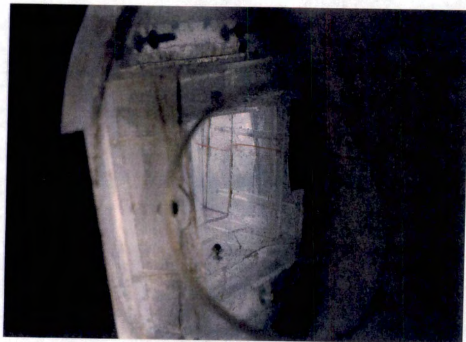
Zone 3, View Upstream into Nozzle Exit
