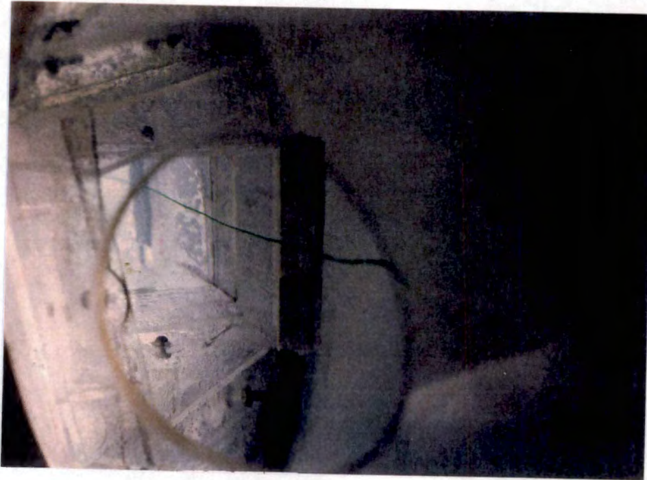
Zone 2, View Upstream into Nozzle Exit
