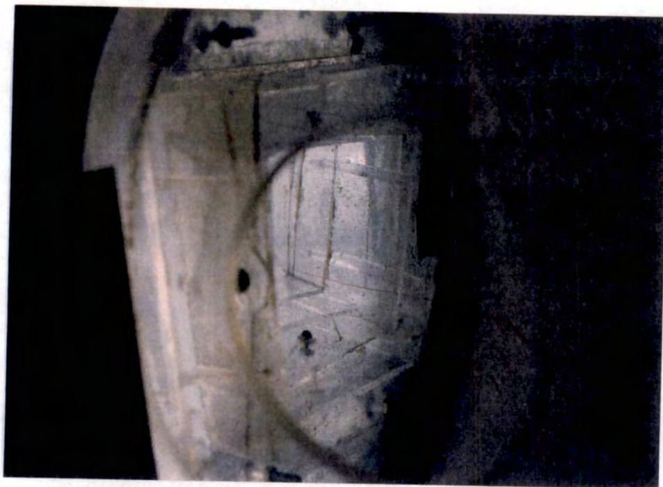
Zone 1, View Upstream into Nozzle Exit
