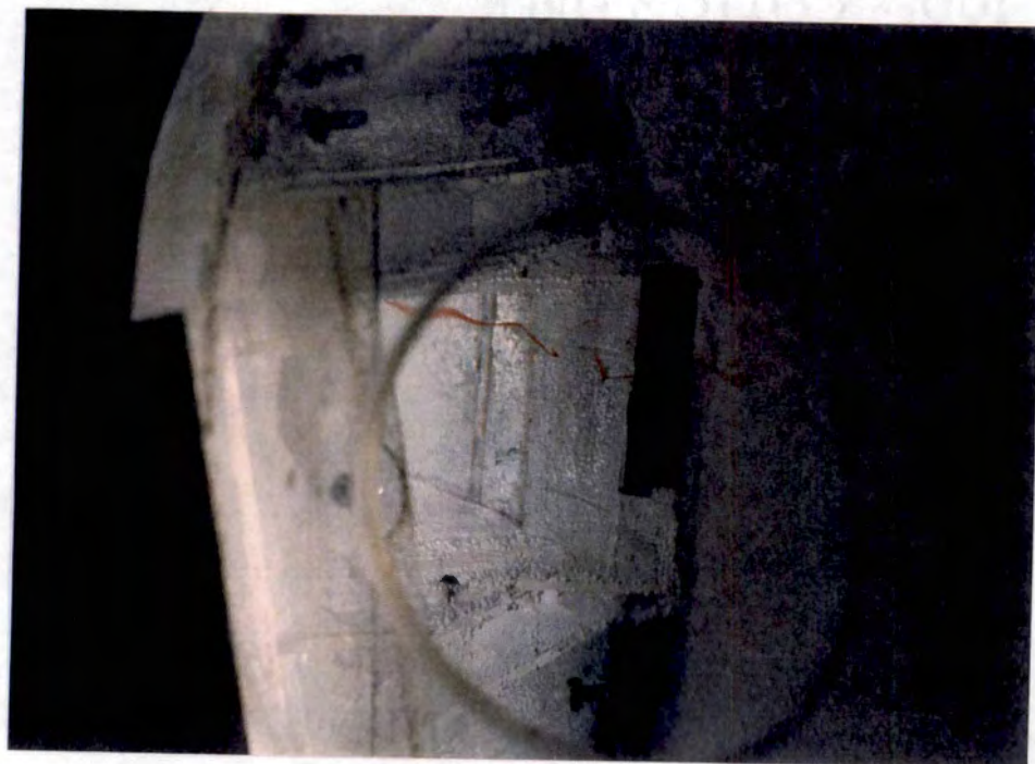
Zone 3, View Upstream into Nozzle Exit
