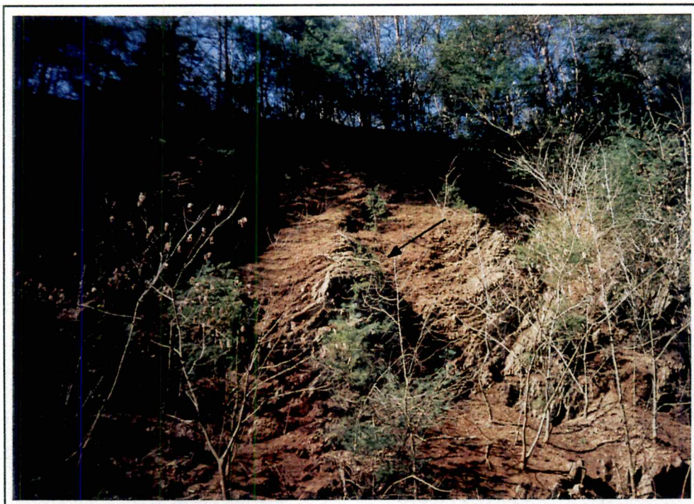
A-3.b Arrow indicates top of the slope cut. The slope at top is highly weathered.
