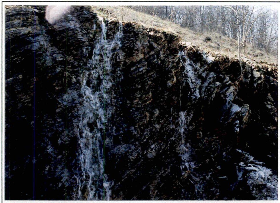
A-1.b The presence of water is one of the factors responsible for the bad conditions of the rock.
