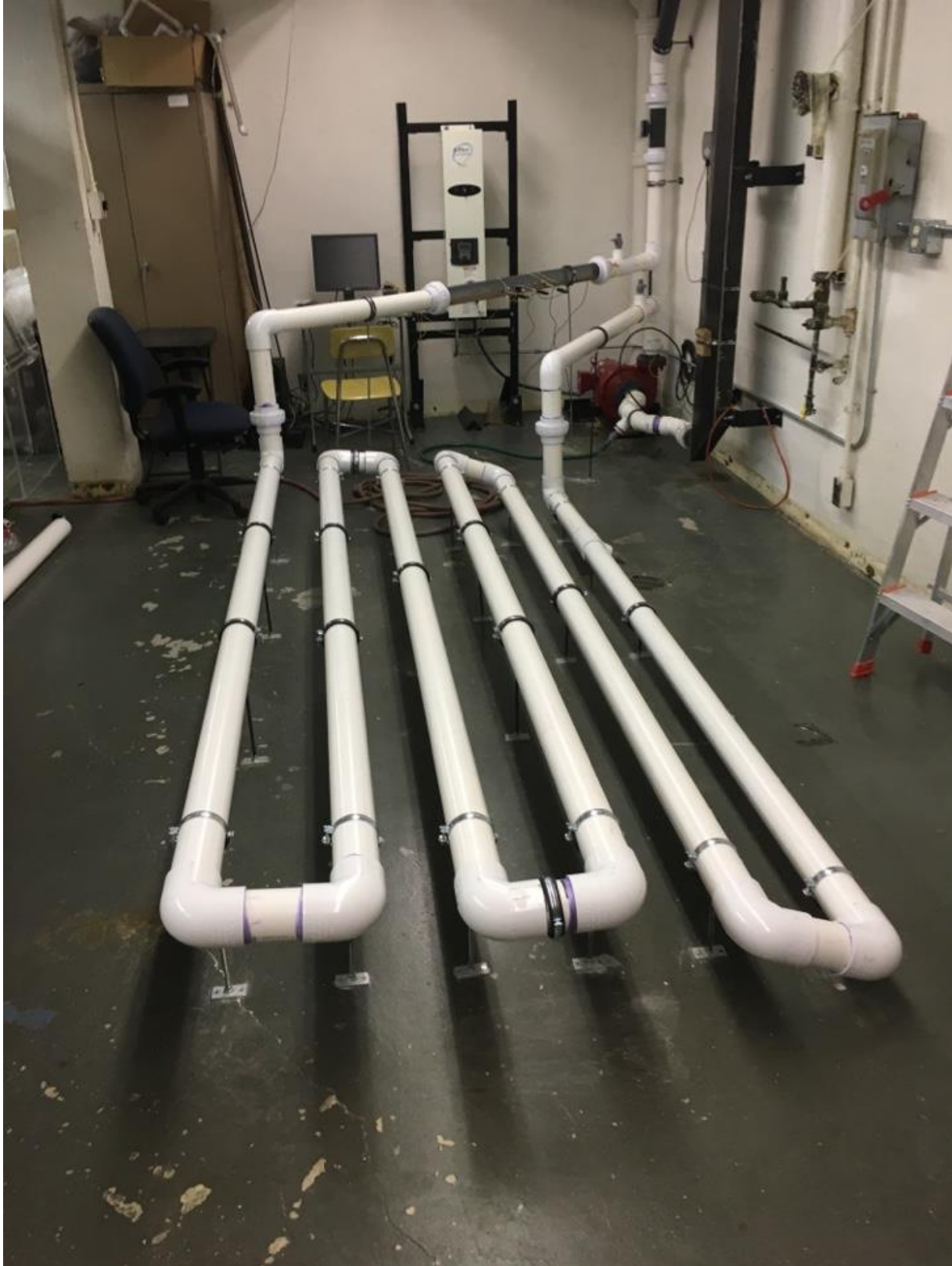
Figure 17: Picture of extra length of piping to stabilize flow and recombine bubbles in flow
