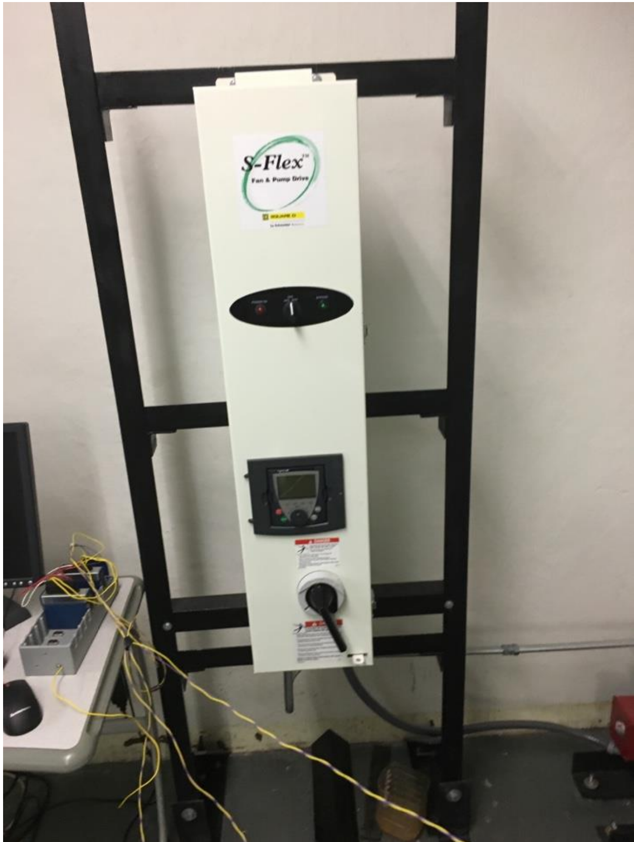
Figure 18: Picture of variable frequency drive
