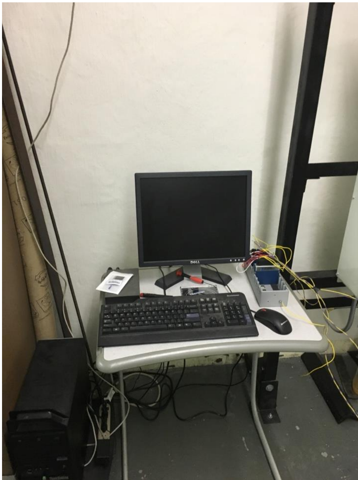
Figure 16: Picture of computer station with DAQ modules on right of desk
