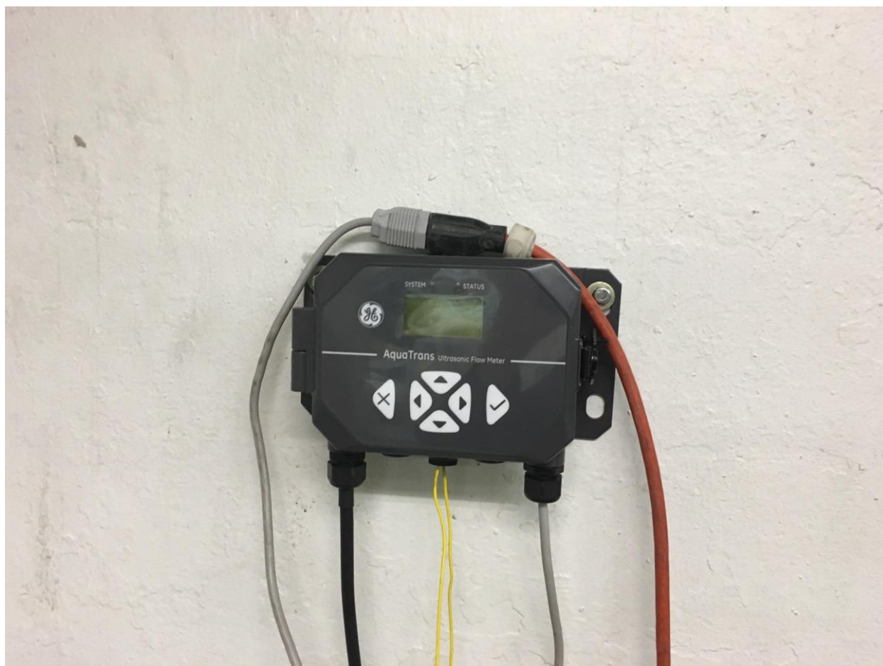
Figure 19: Picture of AT 600 ultrasonic flow meter
