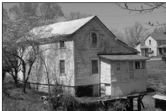
Figure 6.6 Deteriorated housing, Converse, Spartanburg County. March 2004
