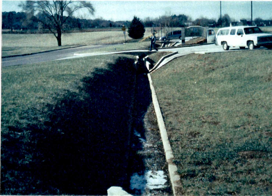
A11.1c - The second pond receives runoff from a parking lot, the first pond, and a pasture. The photograph shows the inlet from the parking lot and the first pond.
