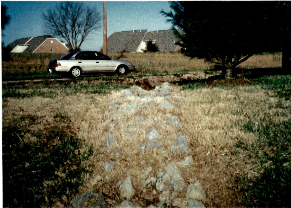
A9.1c - This is a view of the dam and the rip rap emergency spillway. The spillway was designed to be 30 ft. long x 1 ft. deep and 12 ft. to the left of the outlet pipe, but it is actually 3 ft. long x 0.2 ft. deep and directly over the outlet pipe.
