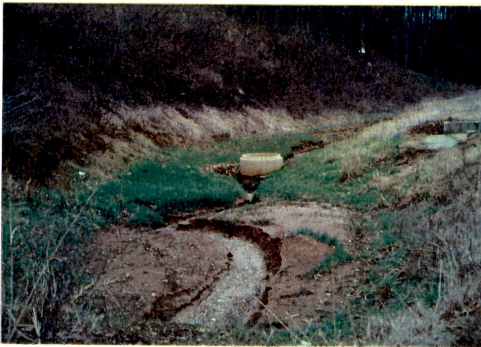
A15.1b - The actual storage volume in the pond is 52% of the intended design storage volume. The net result is that the routed design storm is discharging 3.3 times the pre-development peak flow because the actual water depth is 0.4 ft. higher than the maximum design depth and the water is discharging through the overflow.
