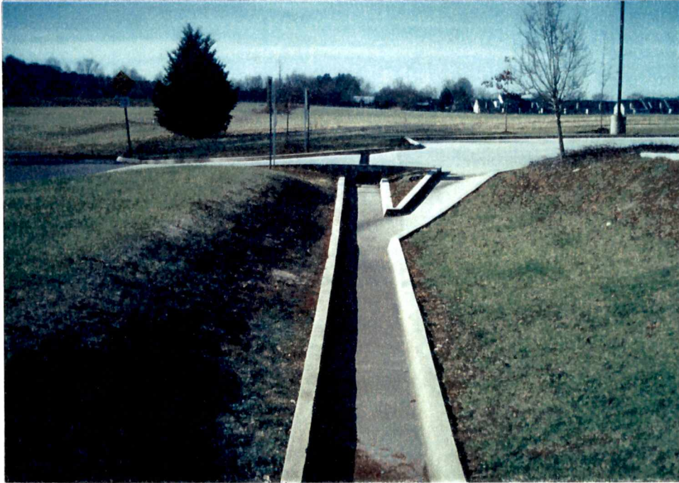
A11.1a - The Pond 11 is divided by an entrance driveway. Therefore, the storage volume is divided between two ponds. This photograph shows the inlet to the first pond. The pond receives runoff from a parking lot.
