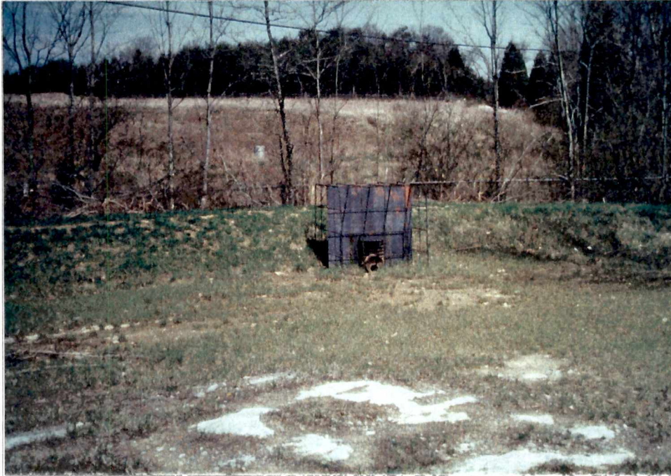
A18.1c - The pond is designed to have 0.43 ac.-ft. of storage volume, but because of bedrock in the bottom of the pond the actual volume is 0.11 ac.-ft. The inadequate storage volume causes a higher water depth during the design storm and the water spills over into the riser, thus exceeding the pre-development flow by a factor of two.
