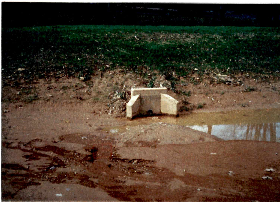
A3.1a - The outlet structure for Pond 3 is a 18 in. diameter CMP having a 6 in. diameter orifice face plate. The pond is filling in with silt from the upstream construction site.
