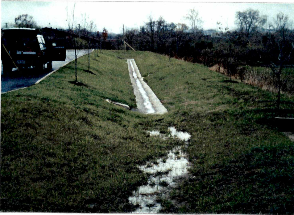
A8.1a - The dam (Right side of photograph) is 2.9 ft. lower than the intended design specified. The routed design storm overtops the dam.
