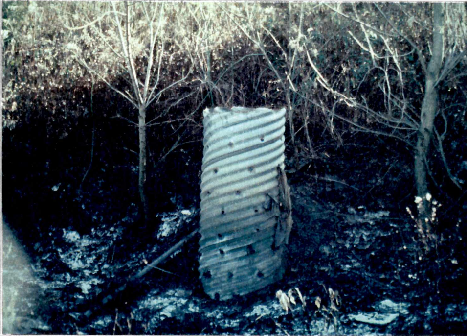
A13.1a - The 18-in. CMP perforated riser pipe is the outlet structure for Pond 13. The perforations are clogged with trash and because, there is no protection on top of the pipe it also has debris and trash in it.
