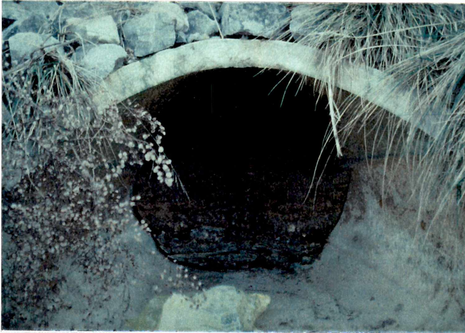
A12.1c - This photograph shows one of the 30 inch diameter plastic inlet pipe to Pond 12. The pipe is half full of mud from the upstream construction. This could have an impact on upstream flow and cause other problems.
