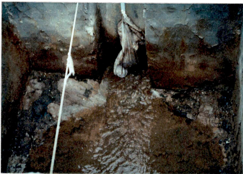
A14.1b - The weir is currently clogged with a plastic bag which is decreasing the discharge capacity.
