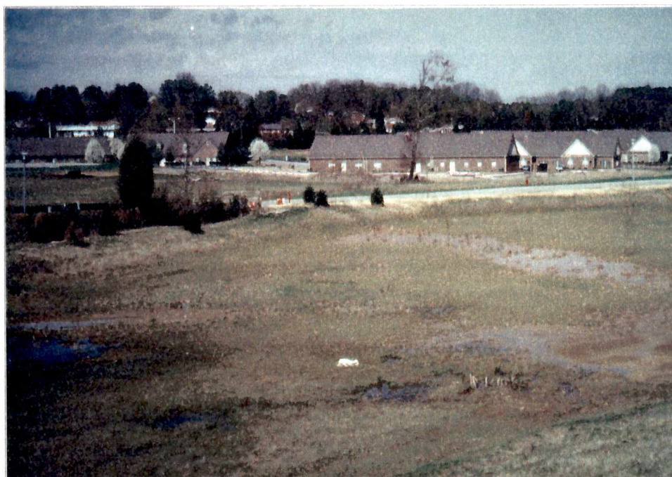
A19.1b -This photograph shows the overall view of the pond. The actual storage volume is only 53% of the intended design volume. The intended storage could not be attained probably due to underlying bedrock.
