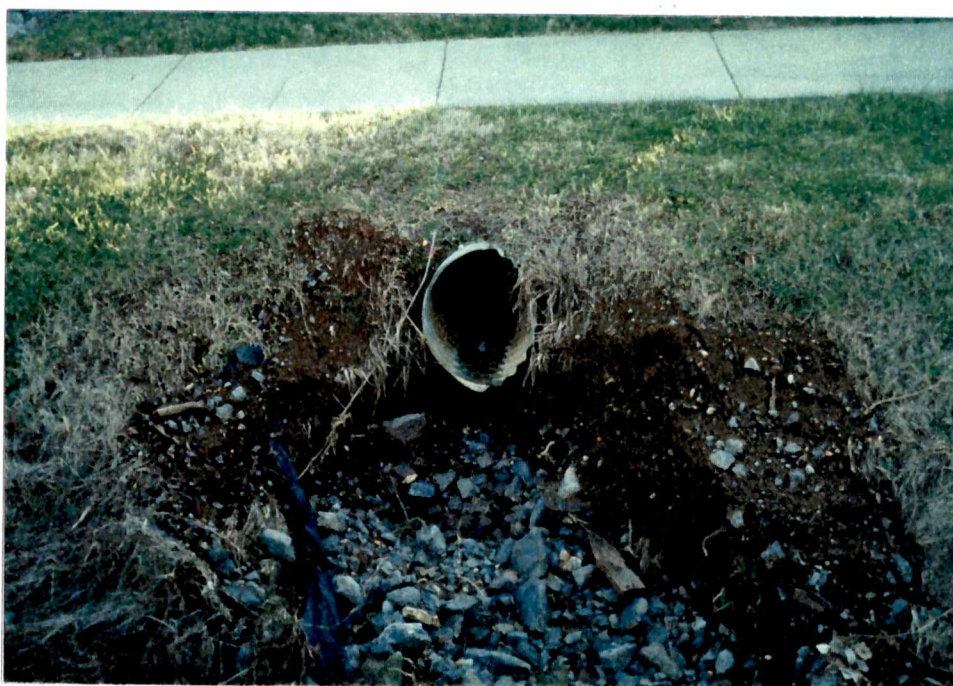
A9.1b - This is the outlet end of the 18-in. diameter CMP. The discharge from the pipe is eroding the side of the ditch.
