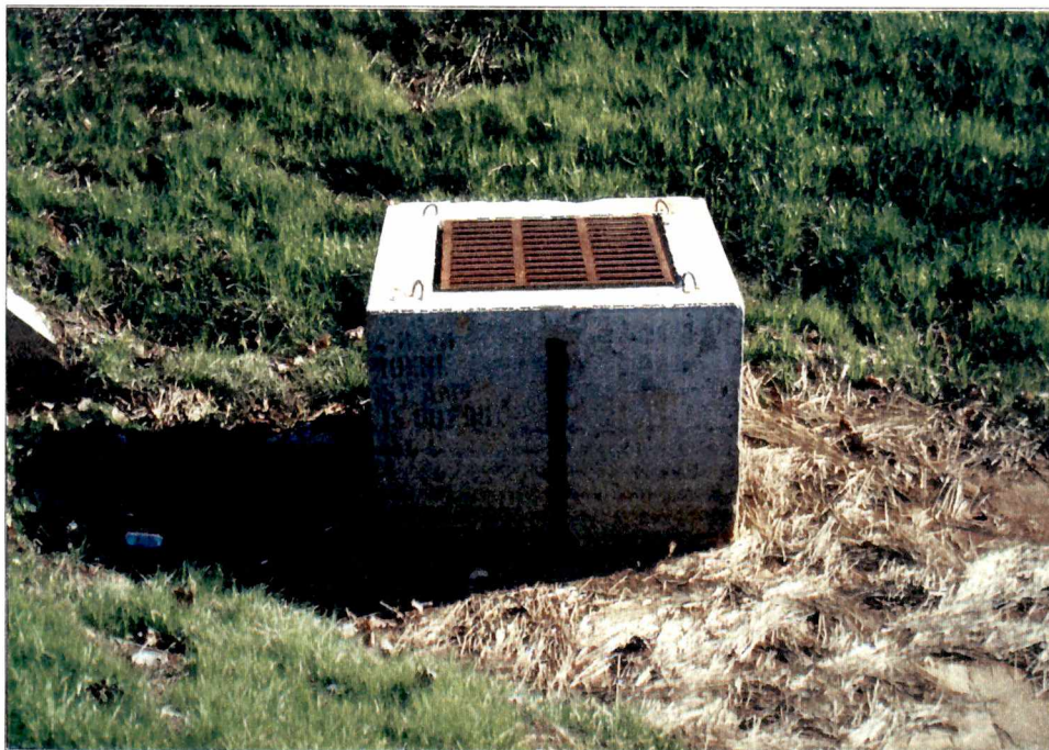
A7.1a - The slot in the outlet structure was designed as a broad crested weir. The slot width was designed to be 0.15 ft. but, it was constructed 0.21 ft. wide.
