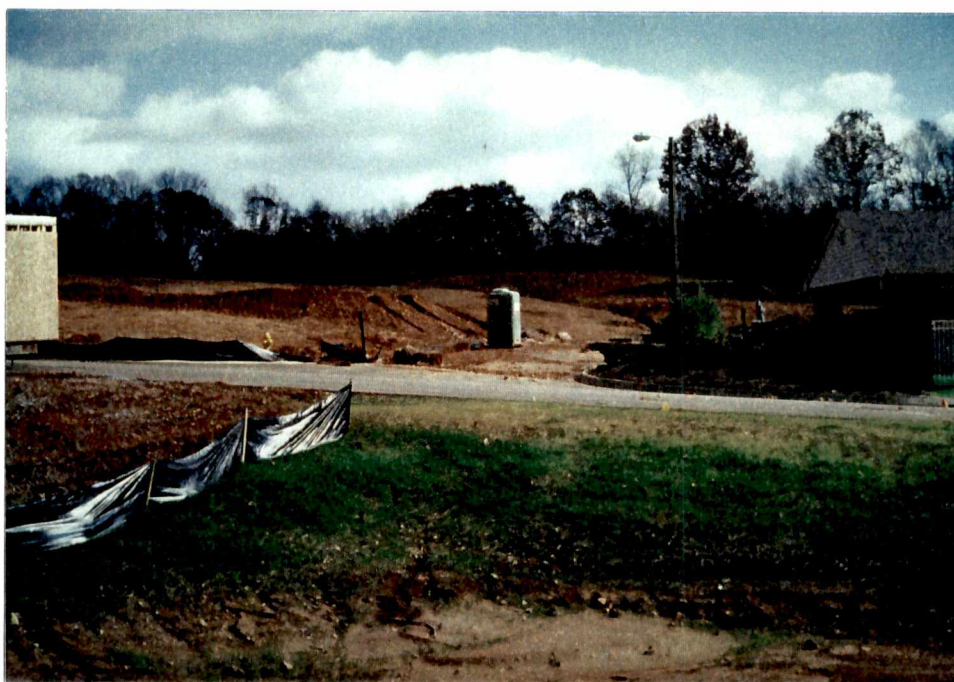
A3.1b - Sediment from this construction site is filling in Pond 3 due to poor erosion control practices.
