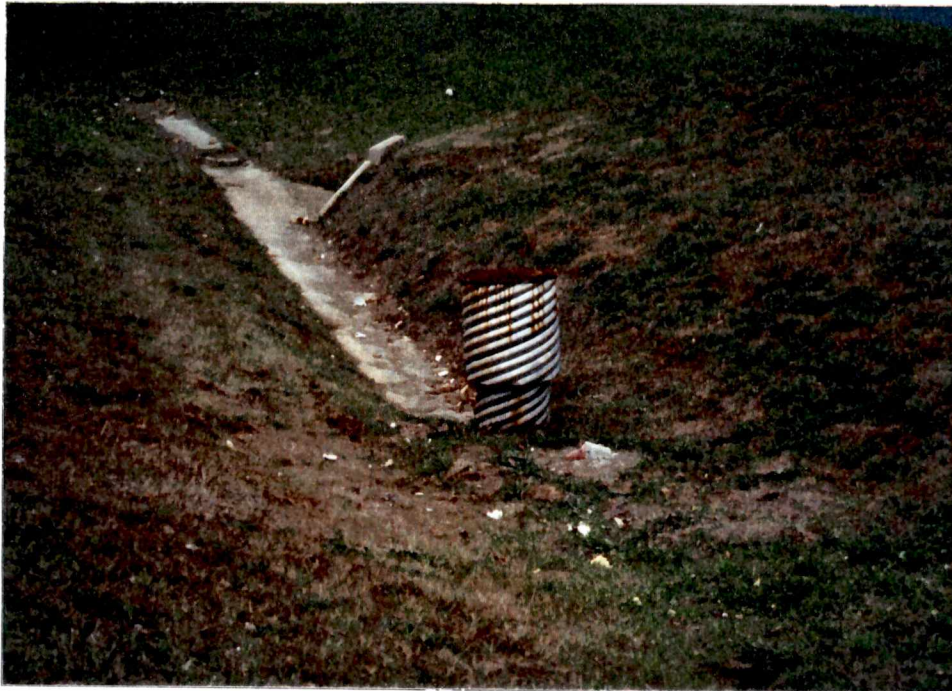
A5.1a - The outlet structure for Pond 5 is an 18-in. diameter CMP riser with a 24-in. diameter CMP anti-vortex device and having a 6-in. diameter CMP at the bottom of the riser. The riser was constructed 1.6 ft. lower than designed.
