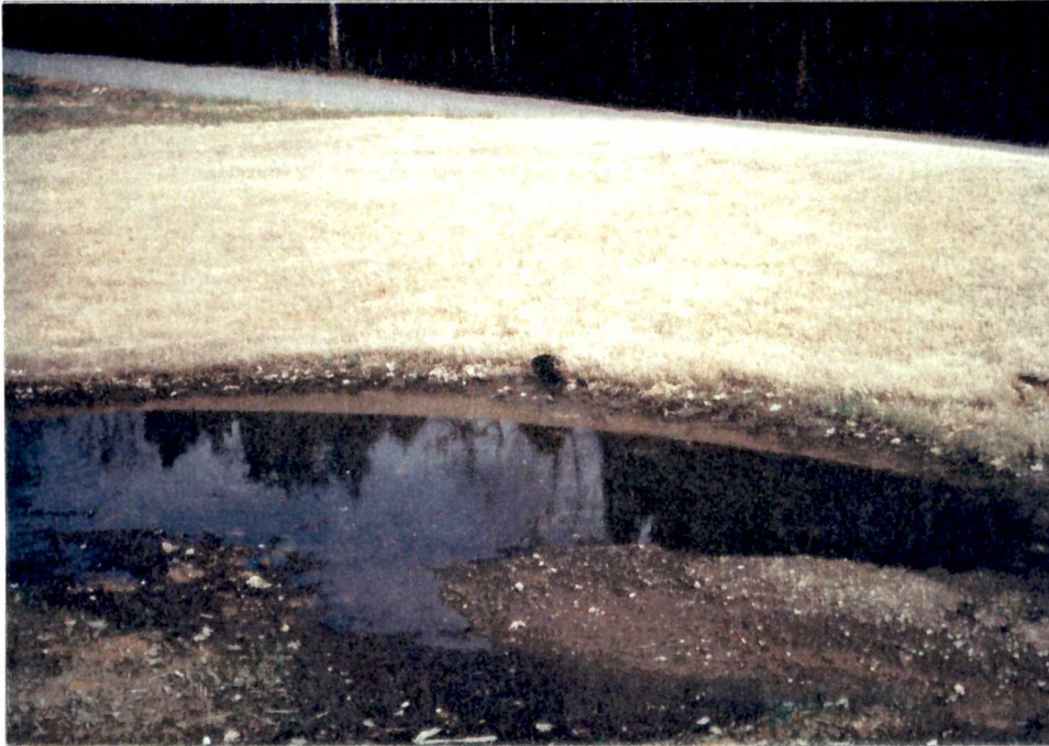
A20.1a - The as-built outlet for Pond 20 is a 15-in. diameter CMP, but a 36-in. diameter riser having an 8-in. diameter riser was the intended design.
