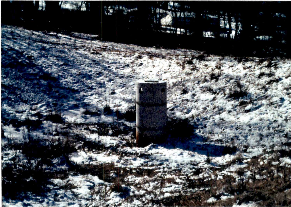
A1.1a - Looking downstream at the outlet structure and dam of Pond 1. The orifice at the bottom of the outlet structure was intended to be a 11.5 in. diameter orifice but, it was constructed as a 10.5 in. diameter orifice.
