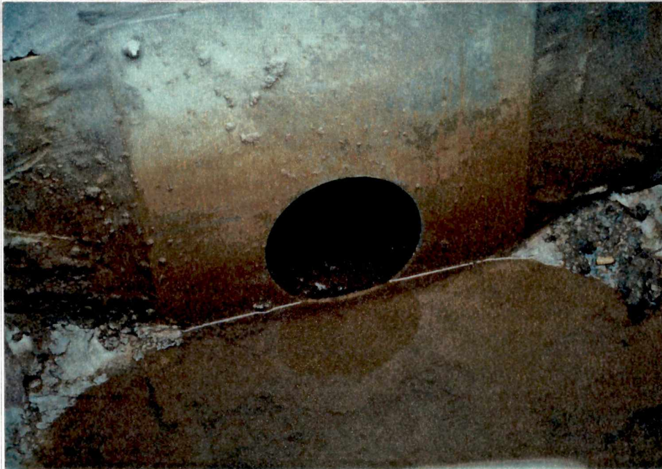
A14.1c - The outlet side of the outlet structure is a 10-in. diameter orifice.
