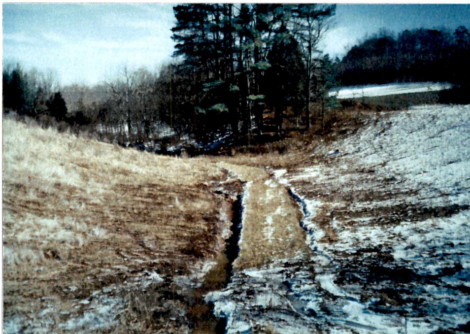
A1.1b - Looking upstream at Pond 1, the area previously wooded, was cleared to build the pond. The bottom of the pond is now eroding into gullies.
