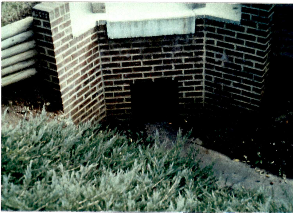
A6.1a - The outlet structure and emergency spillway for Pond 6 was constructed as a 9-in. x 9-in. square orifice but it was intended to be a 9-in. diameter orifice.
