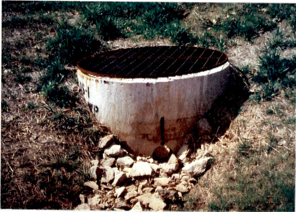
A16.1a - The outlet structure is a 60-in. diameter manhole with a grate on top. The manhole is 2.5 ft. high and has a 7-in. diameter orifice at the bottom. The outlet structure is 1 ft. lower than designed.
