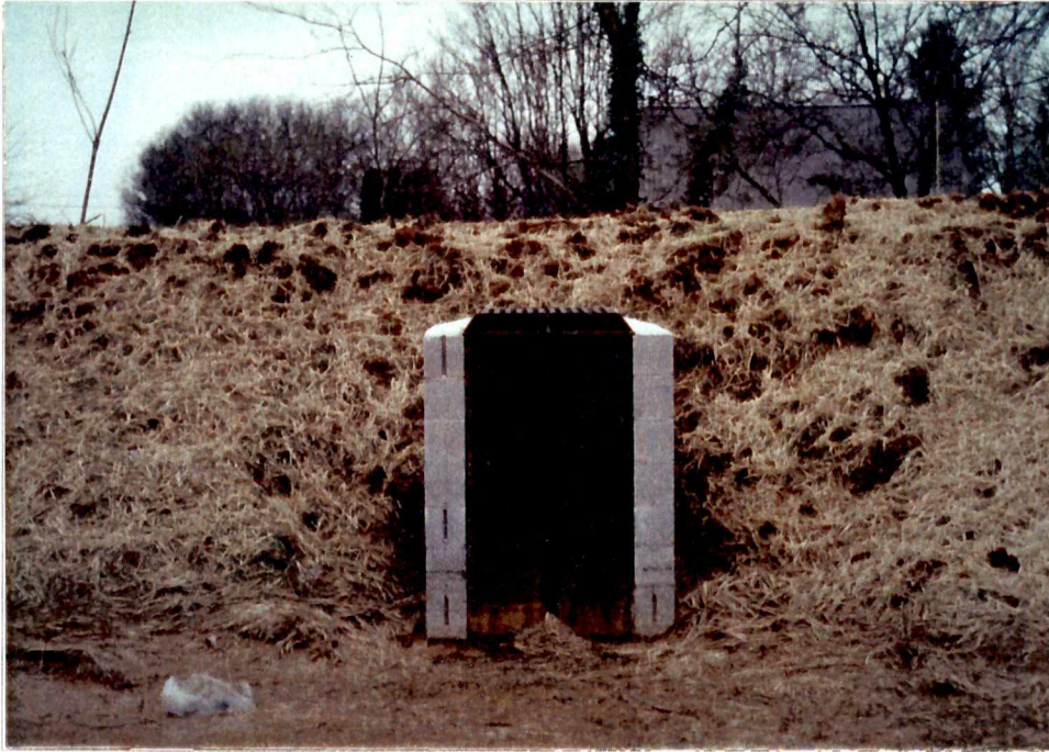
A17.1a - This photograph shows the overall outlet structure and dam. The outlet structure is 0.9 ft. lower than designed. The dam is 0.6 ft. lower than the design plan drawing indicates and is 0.4 ft. higher than the design calculations indicate.
