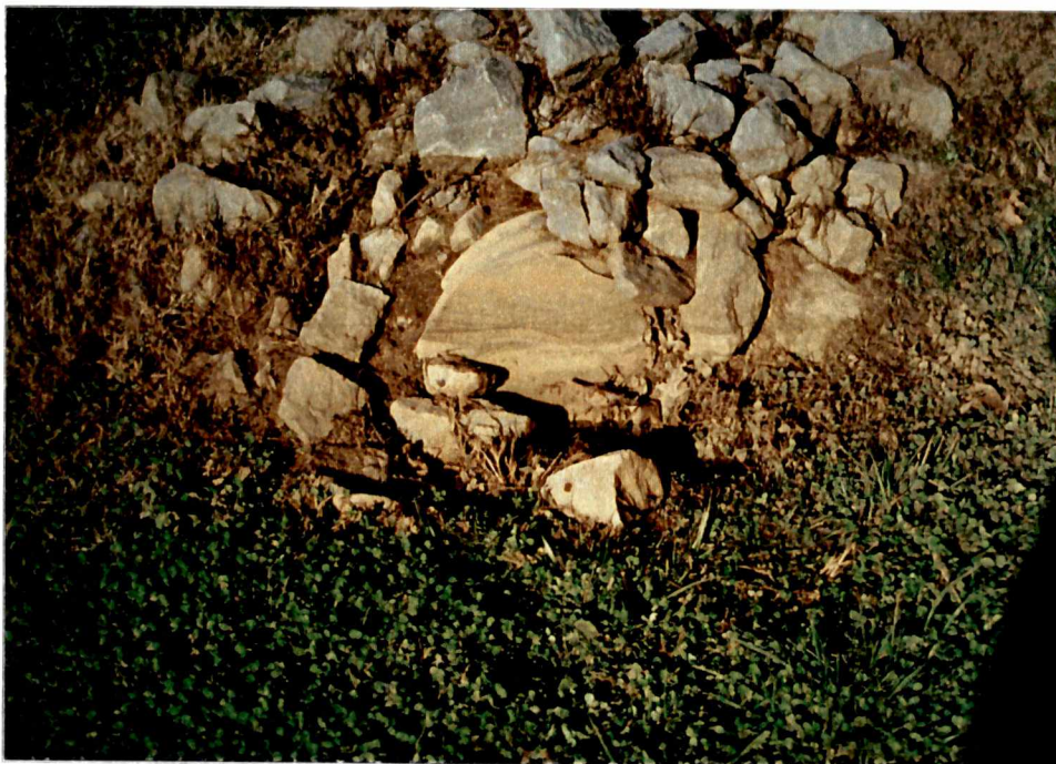
A9.1a - The outlet structure for Pond 9 is an 18-in. diameter CMP having a 5-in. diameter orifice restrictor plate. The orifice was designed as a 12-in. diameter orifice. The orifice is in the center of the photograph in the shaded area.
