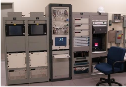
(a). Timing and control center
