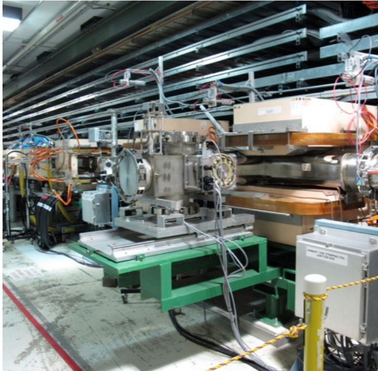
Figure 1.11 - Primary Stripper Foil Changer (PFC). The PFC houses the foils that used within SNS during production.
