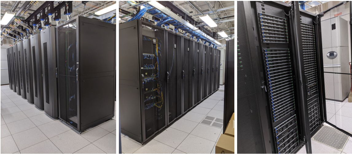
Figure 4.1: ISAAC NG racks front, rear, and server views
