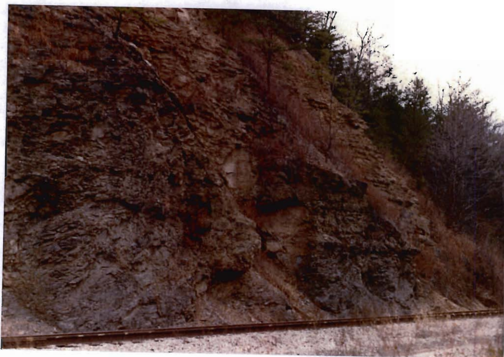
Figure 14. Parallel fractures at Field Station 55.
