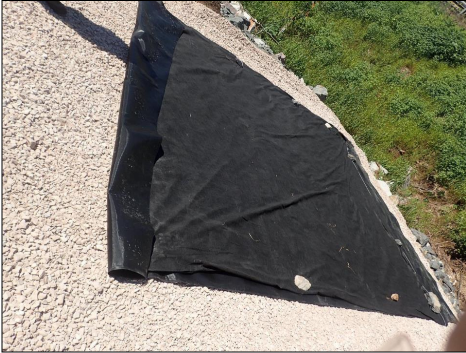
Sediment Filter Bag (EC-STR-2). Pad is ready for a filter bag. It will receive pumped water from suspended pipe diversion.
