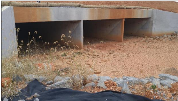
Culvert inlet protection (EC-STR-11A).
