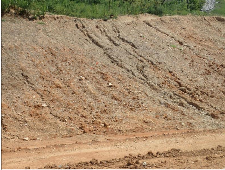
Temporary Slope Stabilization – mulch W/O Seed. Straw is not crimped, light coverage, low berm height failed to divert off site drainage on top of the cut slope. No intermediate protection within the slope.
