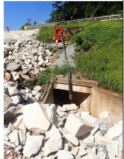
Suspended pipe Diversion (EC-STR-33) Downstream side
