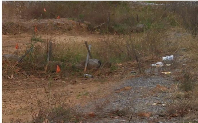
Rock check dam (EC-STR-6) used with sediment tubes (EC-STR-37) for ditch check.
