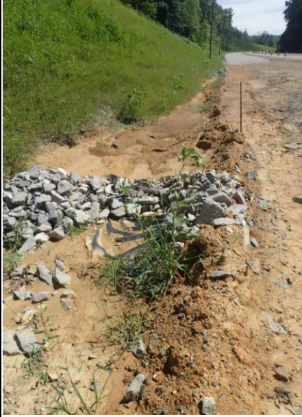
Rock check dam (EC-STR-6) looking upstream
