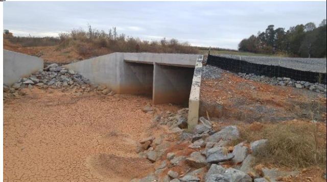
Silt fence with wire backing (EC-STR-3C).
