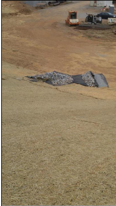
Pipe inlet protection (EC-STR-11) used with Enhanced rock check dam (EC-STR-6A).
