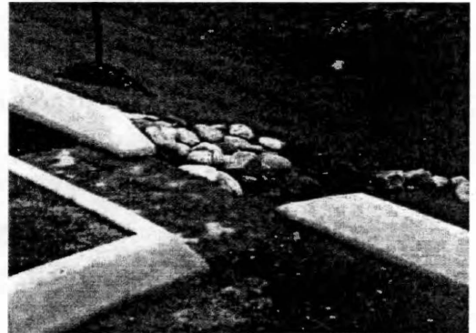
Figure 5.3- Inlet after Failure
