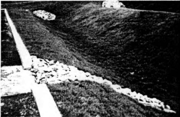
Figure 5.2- Inlet prior to Failure
