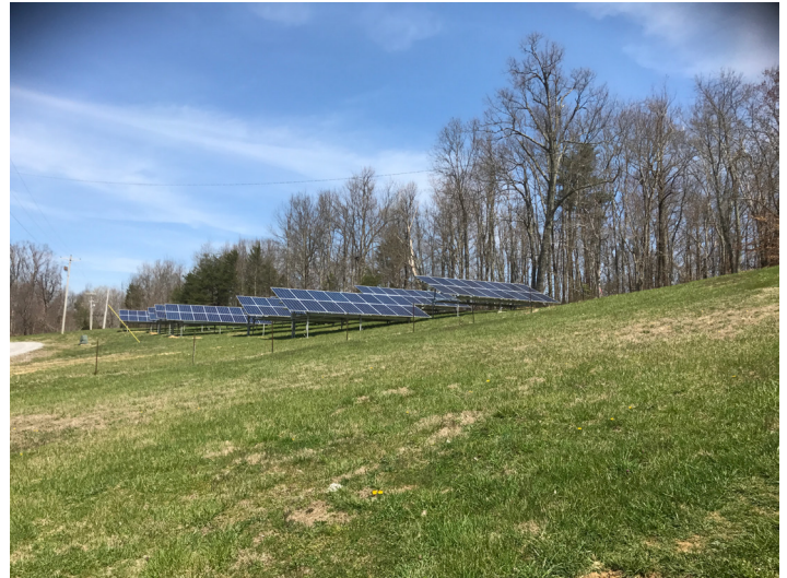
Monterey solar panels
