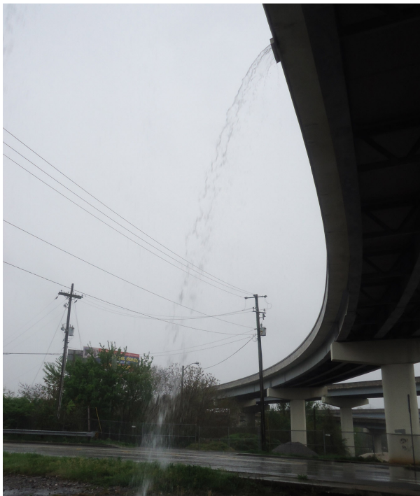
Figure 8. Rainwater falls from the viaduct above.
