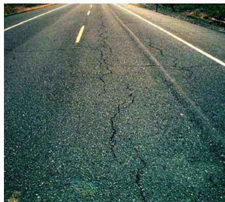
(b) Longitudinal cracking (wheel path)
