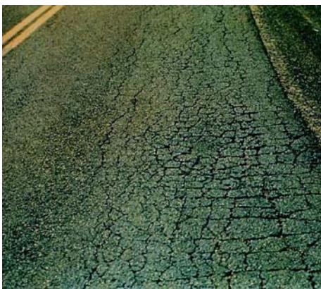
(a) Alligator cracking
