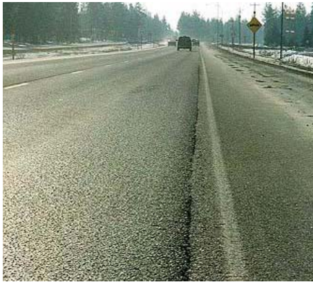
(c) Longitudinal cracking (non-wheel path)
