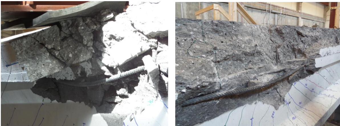
Figure 4.31 – Close up of Damaged Top Flange at Load Point
