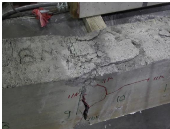
Figure 3.56 – Failure Mode of Specimen A0.62-10
