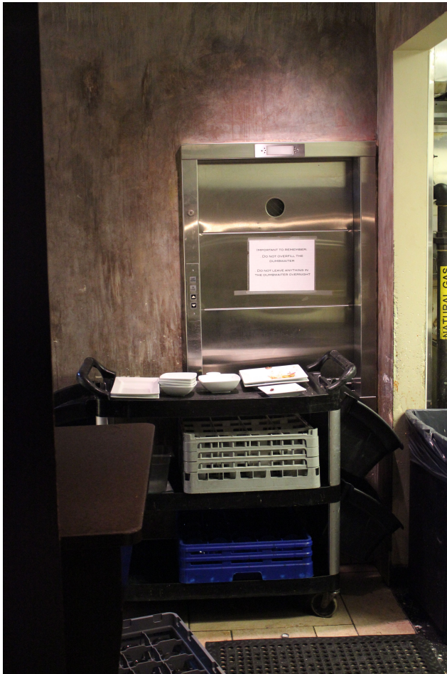
Dumbwaiter used to transport dishes to the basement-level dishwashing station
