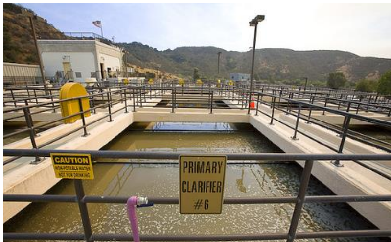
Figure 2. Primary clarifier tank at Hill Canyon WWTP in Ventura County, California. Photo credit: www.greenstockphotos.com
