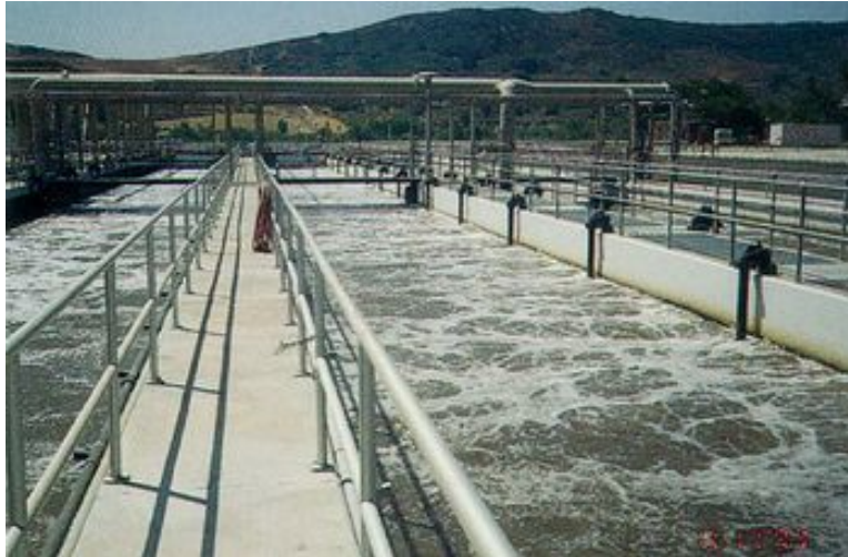
Figure 3. Aeration tank promoting the growth of activated sludge. Photo credit: DCM Process Controls
