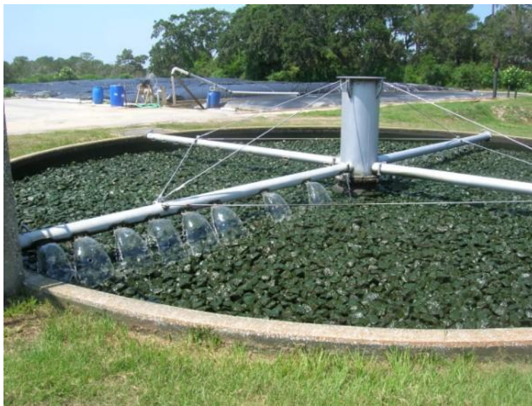
Figure 4. A trickling filter that is evenly discharging wastewater over medium. Photo credit: Utility Compliance INC.
