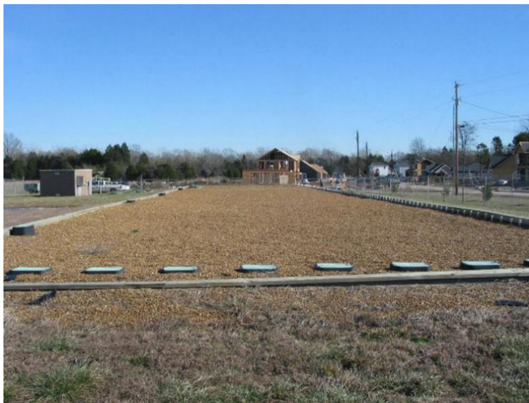
Figure 7. A recirculating media filter located at Murfreesboro, Tennessee, which treats an average 30,000 GPD.
