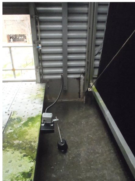
Figure 22 – Float switch inside of the cooling tower's water basin.
