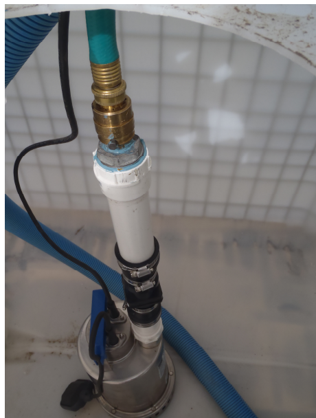
Figure 21 – Submersible pump and check valve inside the storage tank.
