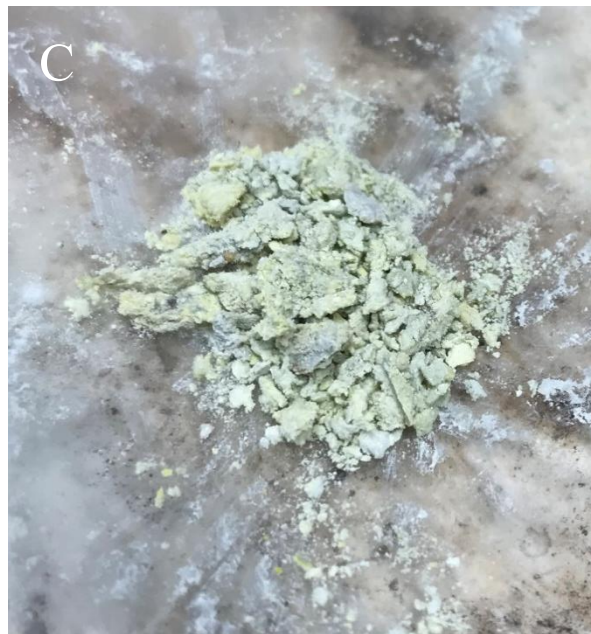
Figure 12. Stages of air exposure to black-purple coating on cladding surface.
