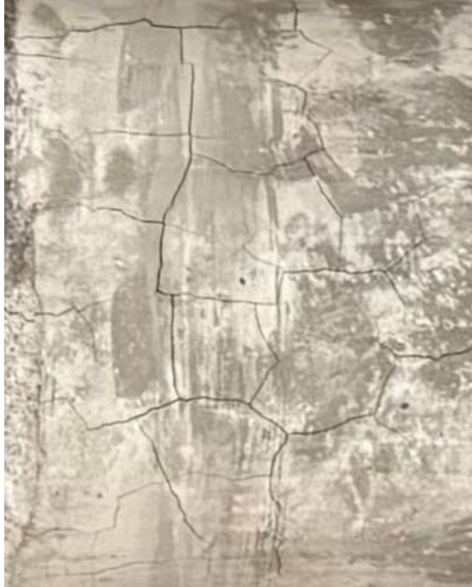
Figure 4-42: Spalled UHPC Surface
