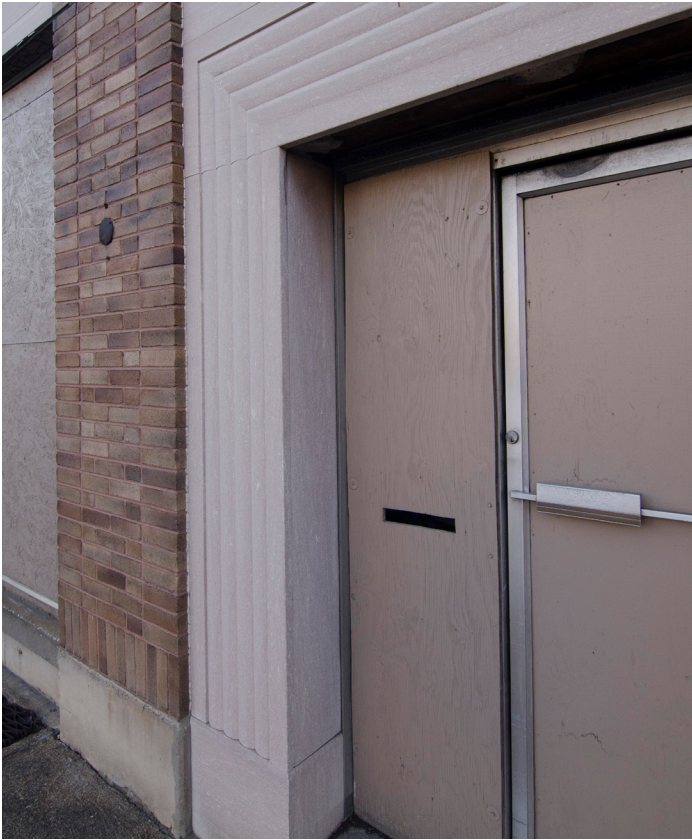
Plywood Prohibits Desirable Transparency of Door
