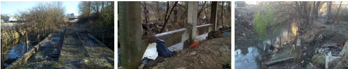
Figure 61: Pictures of debris along 2 nd Creek corridor
