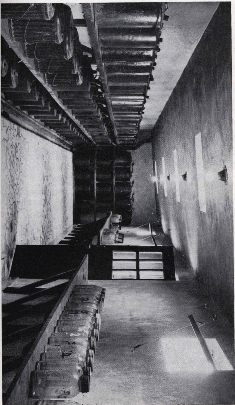
Interior View of the Lysimeter Installation at the Tennessee Station
