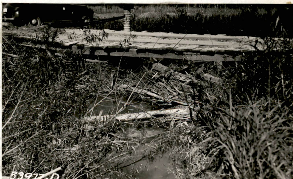
Figure 5. Cane Creek Bridge Blocked by Drift
