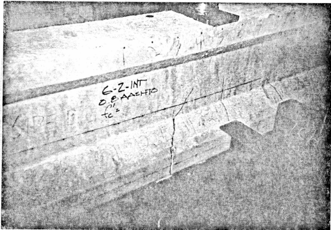
Figure 6.6 Critical Section at Flexural-Shear Crack: Beam 6-2-INT
