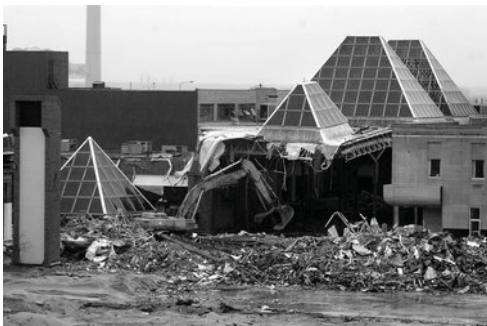
Destruction of Mall
