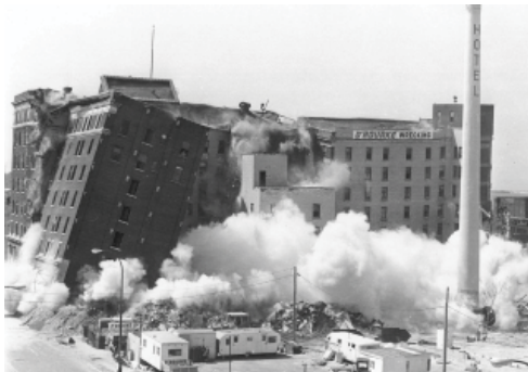
Destruction of Occidental Hotel and other Buildings
