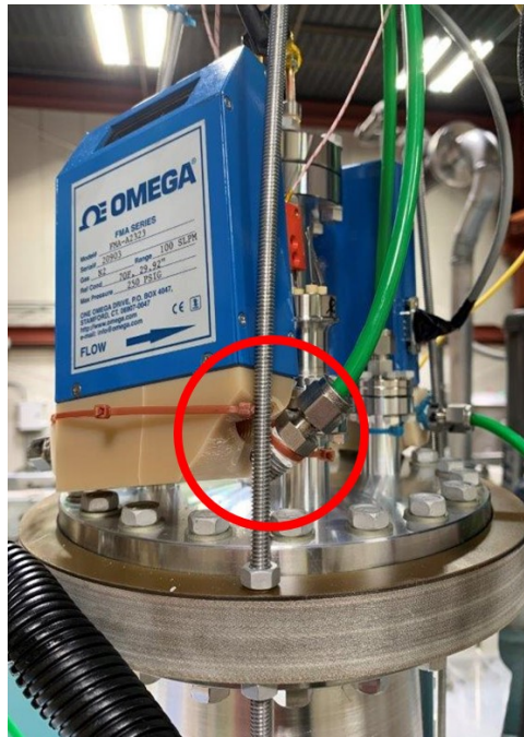
Figure 3.71: Broken flow meter.
